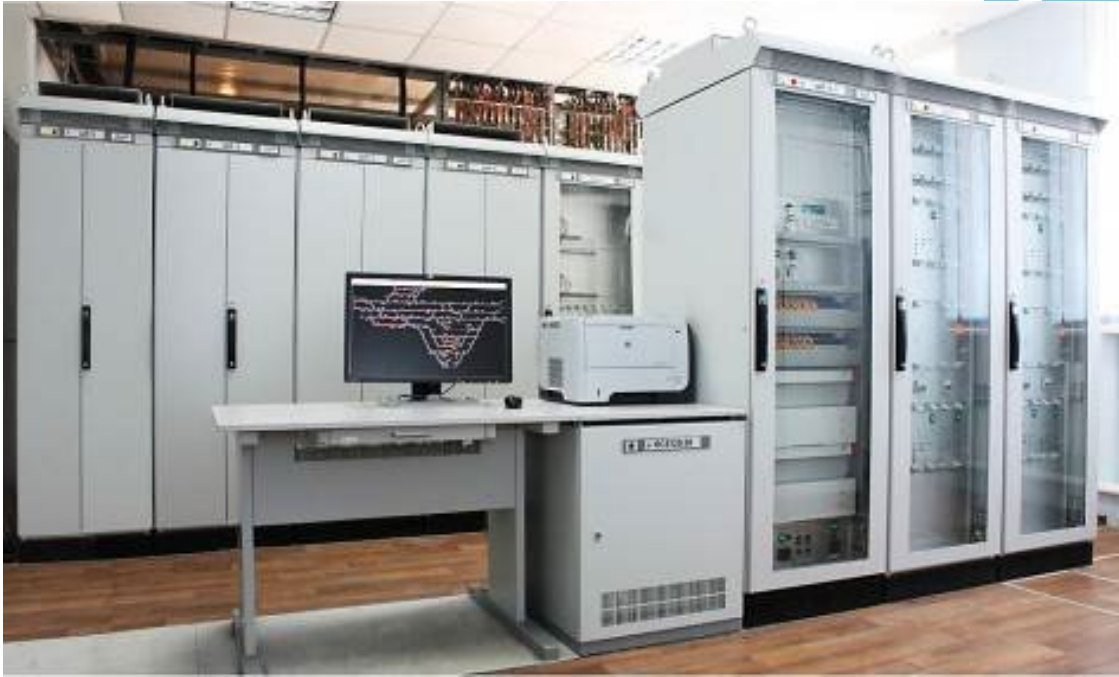
MPC-U at a station (relay room)
