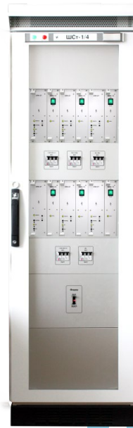
ShSt with battery backup
