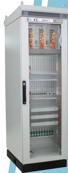
Control cabinet of MPAB-U
